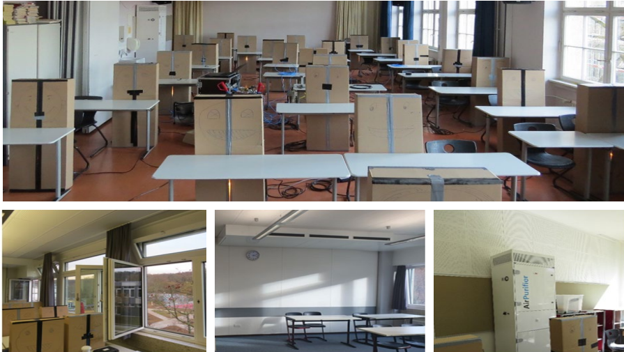
Fig. 8 experimental set up (top), exemplary window ventilation (bottom left), exemplary decentralised ventilation system (bottom middle), exemplary air purifier (bottom right)
