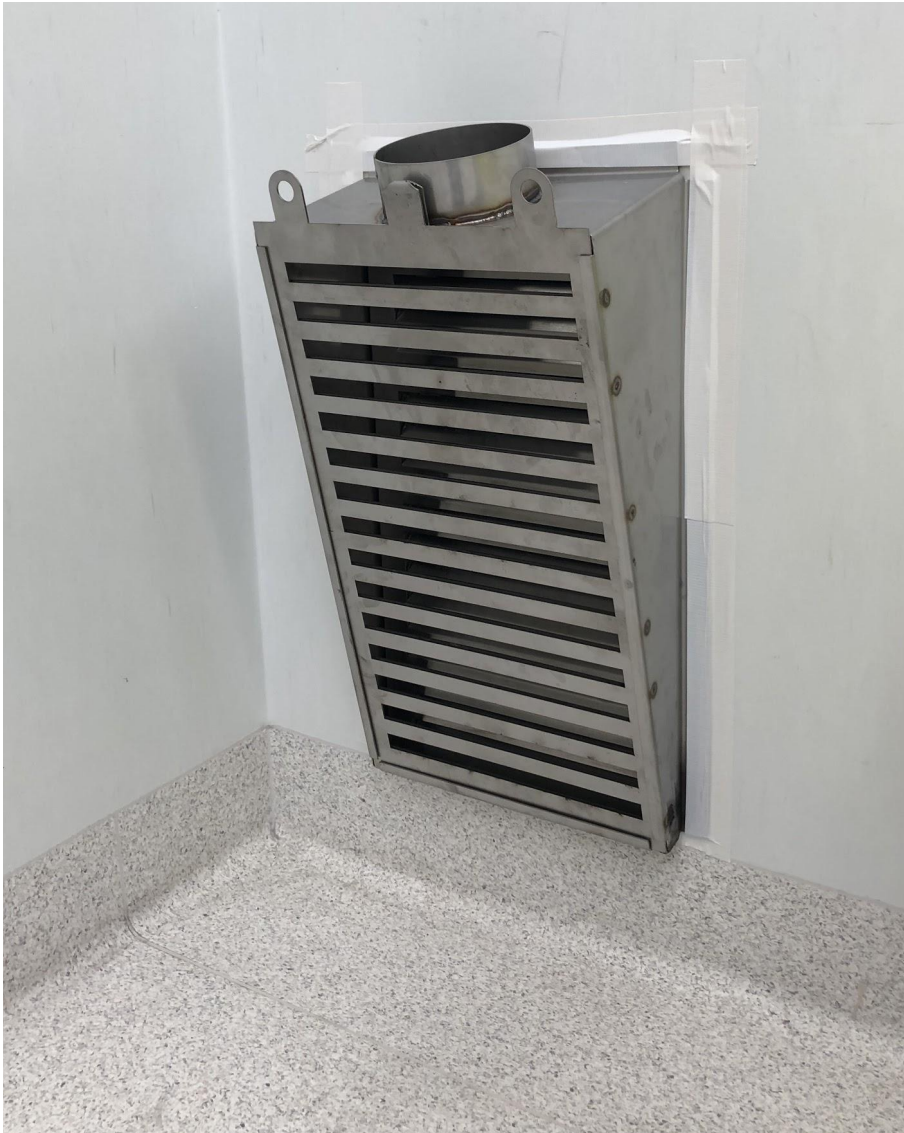
Supplementary Figure 10: Schematic for RIVET Exhaust vent cover version 2.0. Showing sliding louvre system, and hose attachment RIVET Extractor vent cover in situ, affixed to the wall in an airtight yet temporary fashion using duct tape.
